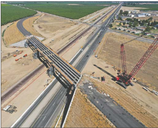
A highway overpass under construction in Merced for California’s planned high-speed rail line from San Francisco to Los Angeles.
