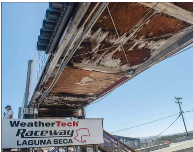
The decrepit start-finish bridge at WeatherTech Raceway Laguna Seca will finally be torn down and replaced with a steel bridge that's ADA accessible and can accommodate carts. The track itself will be resurfaced, as well.
