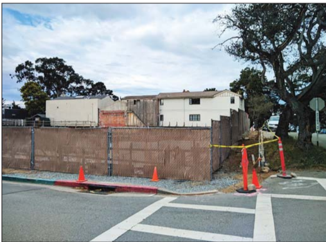
At the urging of public works director Bob Harary, the owners of the construction pit at Dolores and Fifth had workers push back the fencing to free up parking spaces on Fifth and are supposed to build a temporary asphalt sidewalk.
